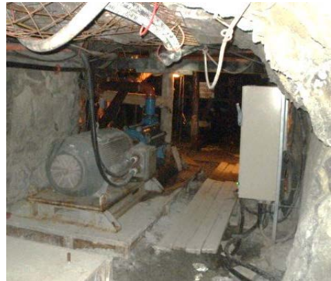
Figure 4 - Lamaque #2 shaft pumping station (475')
