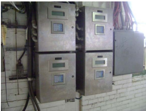
ABB Smart Advisor/Monitoring Technology Corporation P-200/MS-200 Online Vibration Monitoring
