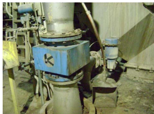
Various Flow Tubes/Valves
