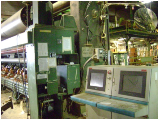
Slitters & ABB Operator Control Stations
