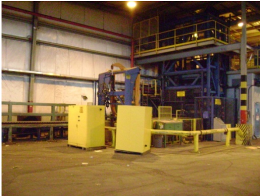
Lamb Roll Upender & Discharge Conveyor
