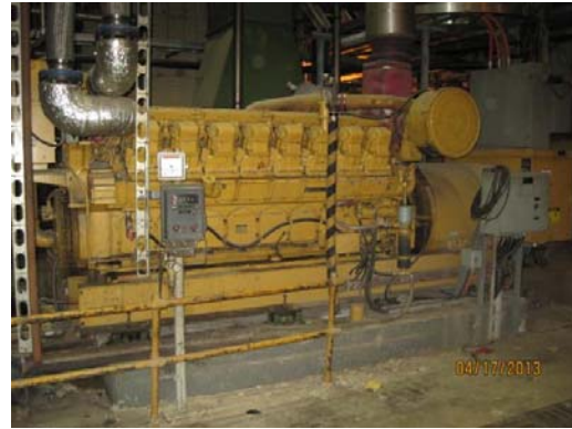
1.5 MW 2400V Diesel Generator
