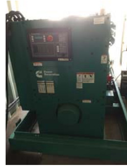
Cummins Diesel Generator QSX15 Litre
