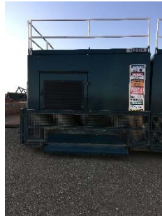
3.5A Mud Pump Building #1
