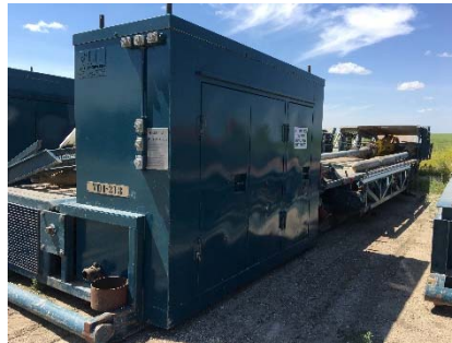
1.8 Catwalk and Manifold Shack
