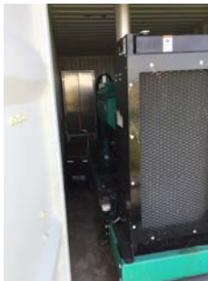
Cummins Diesel Generator QSX15 Litre
