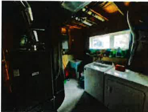
Typical Mechanical / Laundry Room
