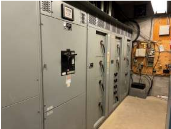
Subject Improvements – Mechanicals
