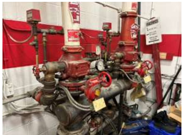
Subject Improvements – Mechanicals
