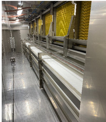
Inside Tunnel Freezer
