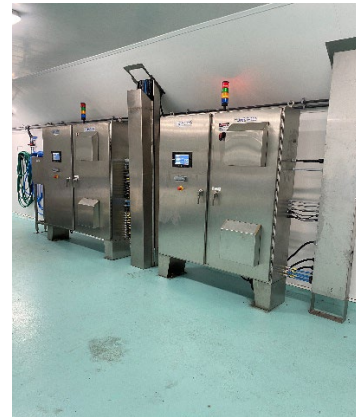
JRT Omron Control Panels
