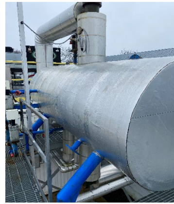
Low Pressure Receiver Tank Tunnel Freezer Refrigeration
