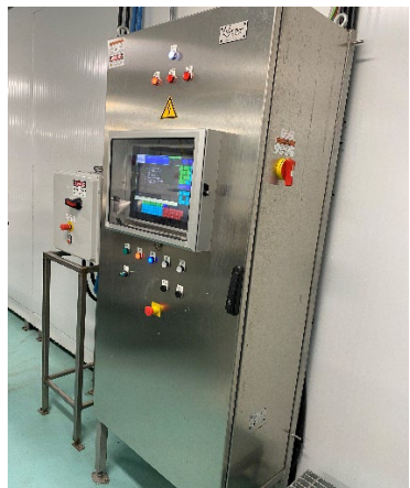
Processing Line Control Panel
