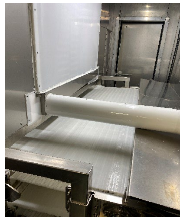
Inside Tunnel Freezer Glazer
