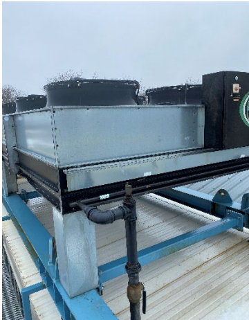
Roof Top Condenser Units
