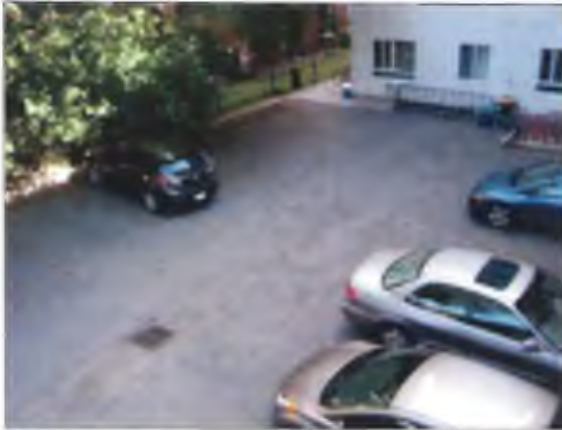
View of the east portion of the asphalt surfaced parking area on the north portion of the Site.
