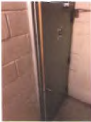
345 – stairwell door not closing
