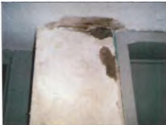
View of damaged plaster within the 7 th floor corridor.
