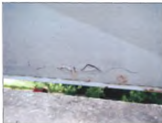
View of minor corrosion on a balcony privacy panel.
