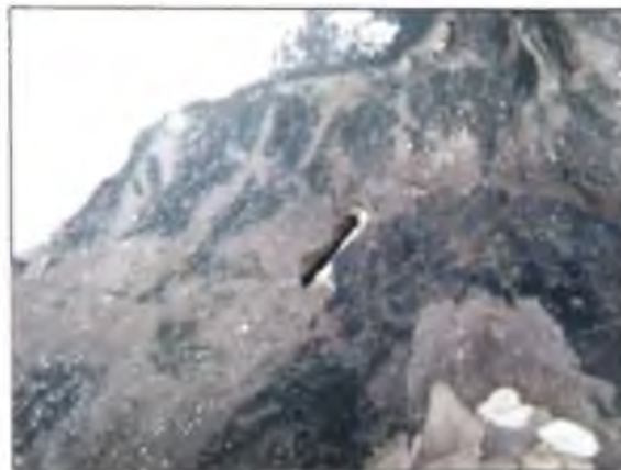
View of an opening in the perimeter membrane flashing at the stairwell penthouse.
