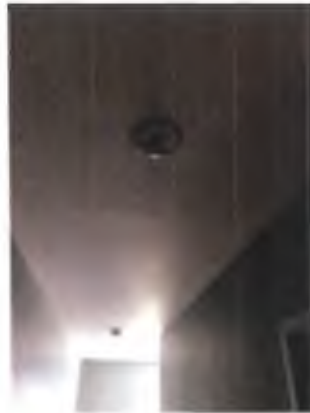
347 – missing smoke detector
