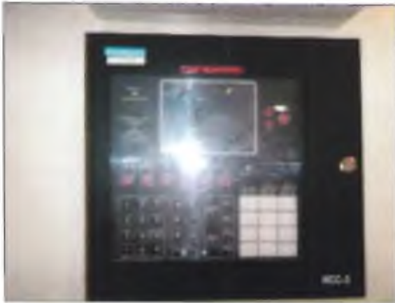
View of the fire alarm annunciator panel within the addition of the Site Building.
