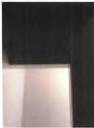
345 – burnt out exit light
