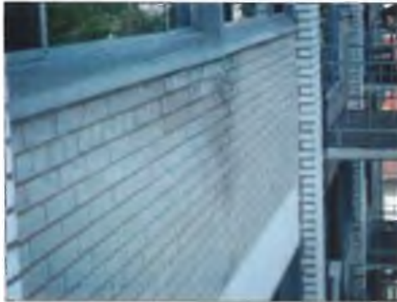
Additional view of the delaminated brick noted from the balcony of unit 707.
