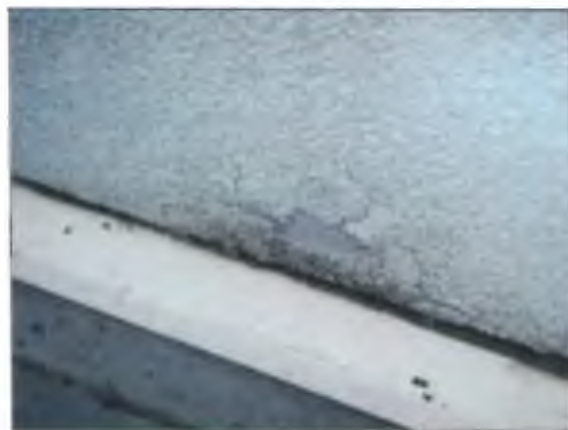
View of cracking in the base of the EIFS on the north elevation.
