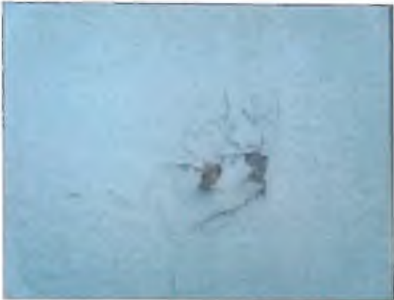
View of delaminated paint on the stairwell penthouse.
