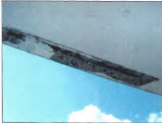
View of a delaminated slab edge at unit 501.
