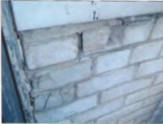
View of the delaminated brick noted from the balcony of unit 707.
