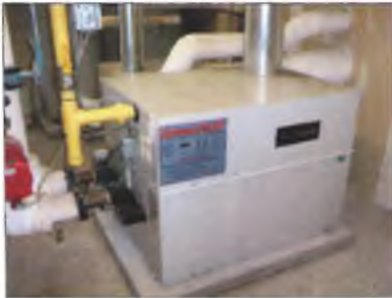
View of the heating boilers within the 2007 addition.
