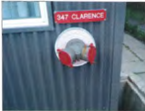
View of the fire department connection at the 2007 addition.
