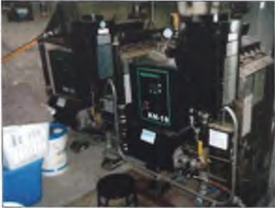
View of the boilers within the original portion of the Site Building.
