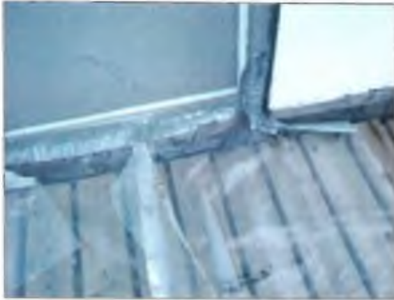
View of polyethylene sheeting installed at the entrance of the stairwell penthouse.
