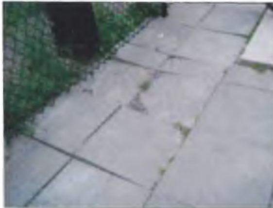
View of settlement of the precast concrete unit paving stones on the north portion of the Site.
