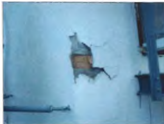
View of delaminated parging and brick noted on the stairwell penthouse.
