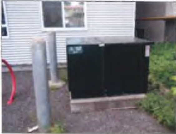
View of the pad mounted transformer which serves the addition portion of the Site Building.
