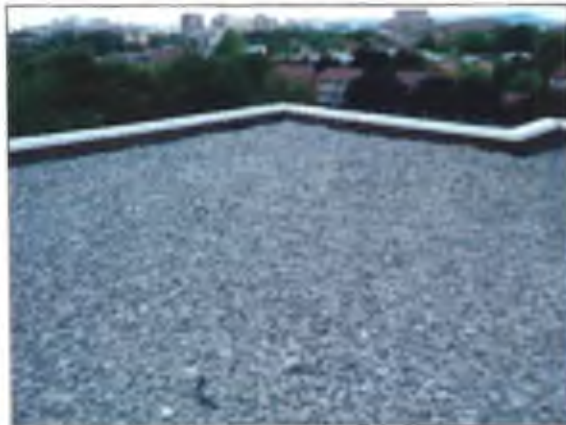
View of the IRMA system atop the addition portion of the Site Building.
