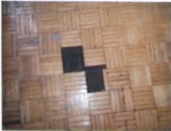
View of damaged parquet wood flooring within a residential unit.
