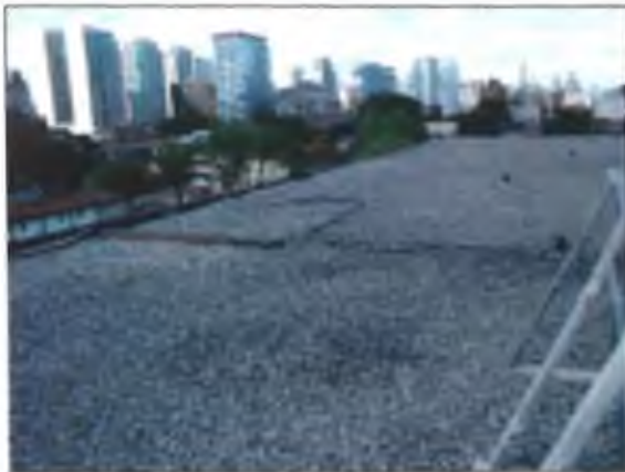
View of the IRMA system atop the original portion of the Site Building.
