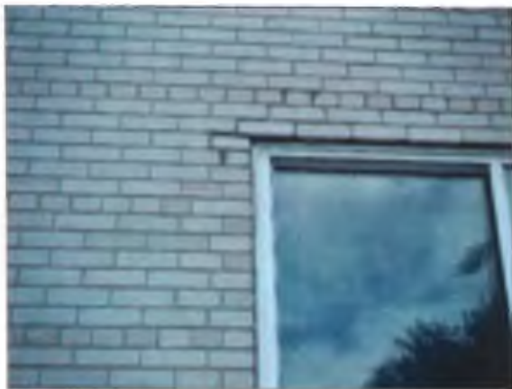
View of delaminated brick noted on the east elevation.
