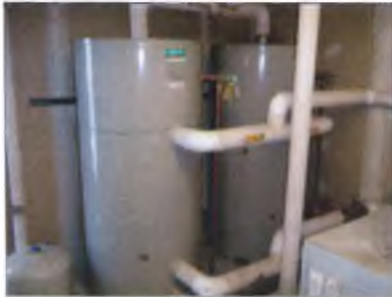
View of the DHW storage tanks within the 2007 addition.
