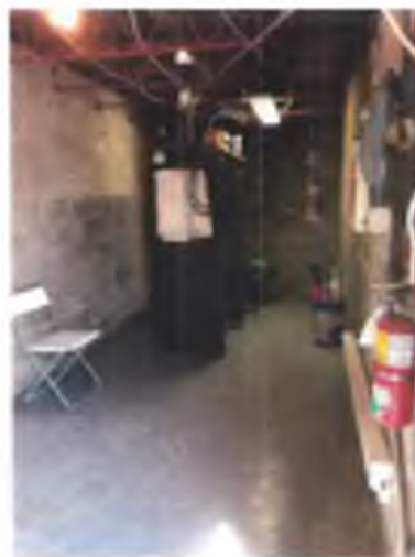
345 – elevator mechanical room
