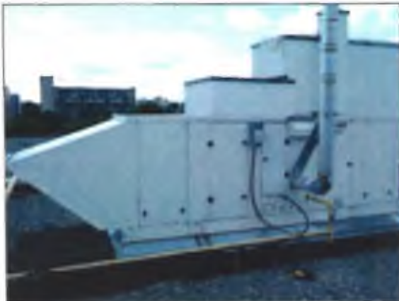
View of the MUA unit atop the 2007 addition.
