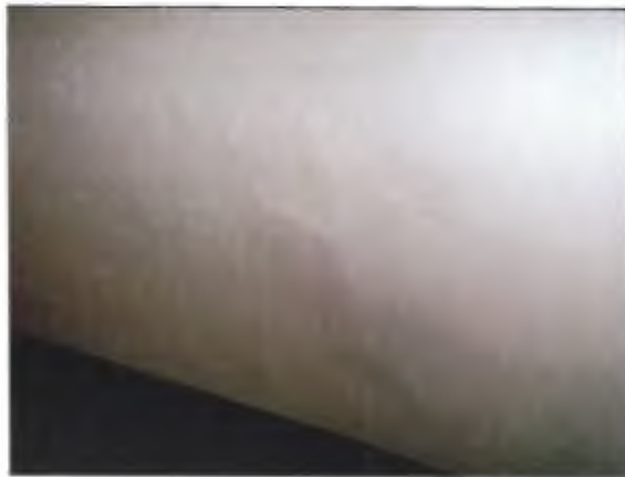
View of an area of plaster popping within the 2 nd floor level.
