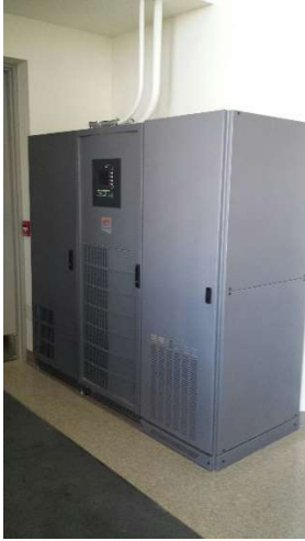
#89 Uninterruptible Power Supply APC
