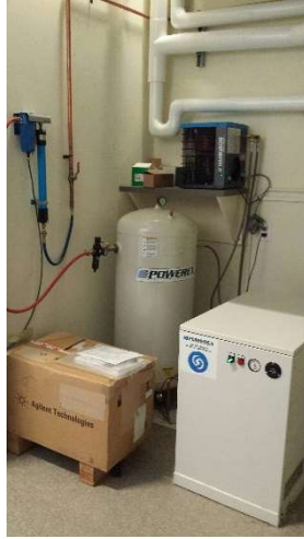
#90 Compressor with Dryer System
