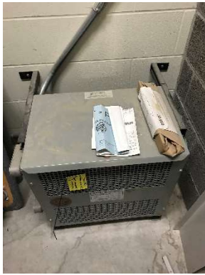
#1 Transformer 600/480V 30kVA
