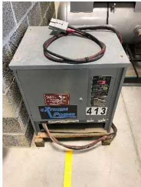
#4 Forklift Battery Charger
